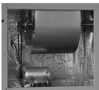
Figure 2. Belt drive motor
